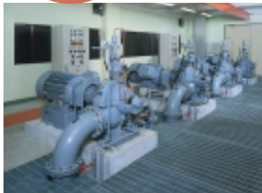
High-efficiency pump flow control
