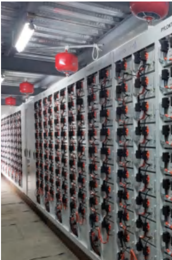
BEIJING CHINA 2.65MWH/1.2MW Micro-grid Self-consumption /Back-up ESS PV+DG+BESS
