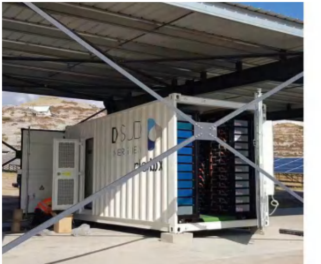
MADAGASCAR 1.5MWH/500KW Micro-grid Self-consumption ESS PV+DG+BESS
